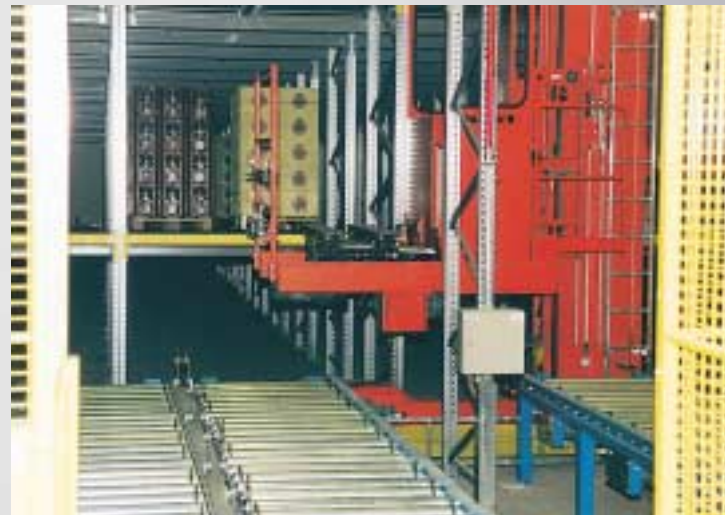
Buffer conveyor at receiving, Storage and retrieval unit, Putting into dynamic storage
