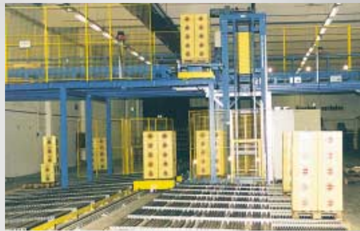
Pallet transport, linking dynamic storage with the commissioning zone
