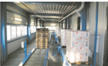
The high-rise warehouse is linked to the palleting facility by connecting bridges.
